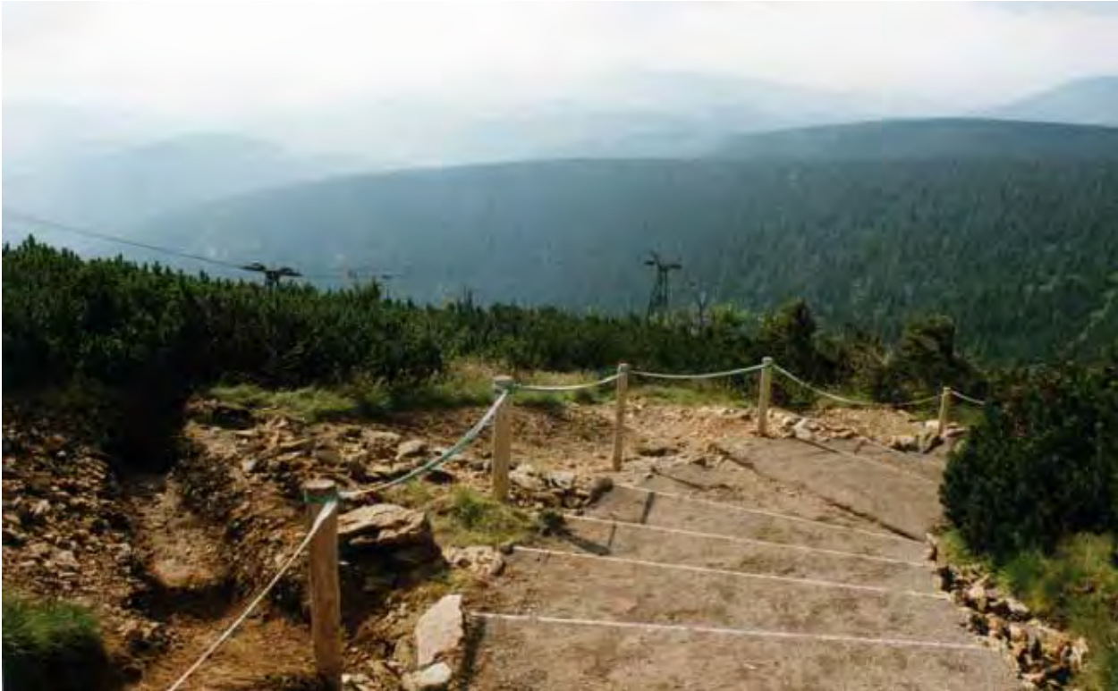
The system of transverse kerbstones and lateral drainage trenches prevents the erosion of construction materials from the pavement, by reducing the erosive strength of the surface water after heavy rain or from melting snow. However, regular maintenance work by the mountain trail builders is necessary to keep the pavement in good condition (photo Jan Štursa)
