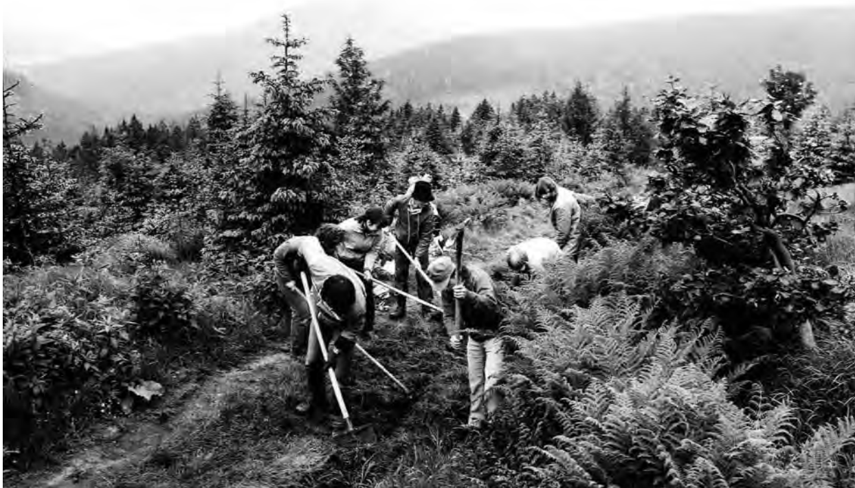
'Young Hands for Krkonoše' event – repairing the trail and its drainage between the Martinova and Labská bouda Chalets, 1984 (photo Jiří Bruník)
