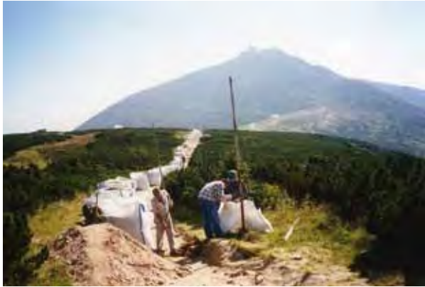
Sacks containing the remaining hundreds of tonnes of limestone from the trail from the Úpské rašeliniště Peatbog below Mt. Sněžka were removed by helicopter. This demanding reconstruction in 2001 was financed by the Ministry of the Environment from the Landscape Care Programme (photo Jan Štursa)
