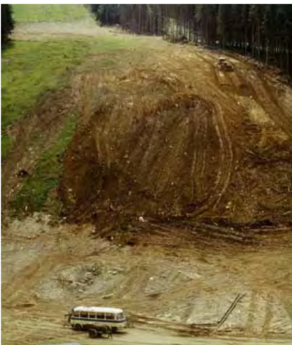
Insufficiently stabilised slope of the 'Great Drum' on the black ski slope at Svatý Petr during modifications in the 1970s (photo Jan Štursa)
