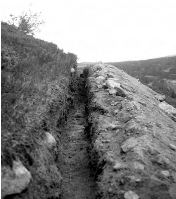
The badly-chosen route for the trench carrying waste from the biological septic tank at the new Labská bouda Chalet led directly into strictly protected Navorská jáma Cirque. The mistake was corrected in time and the trench was backfilled and restored to nature (photo Jan Štursa)
