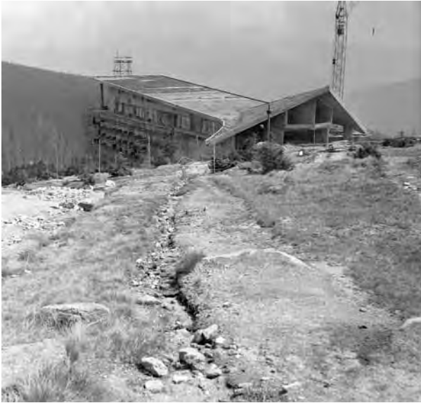
Damage to the terrain along the route of the water mains to the new Labská bouda Chalet (photo Jan Štursa)
