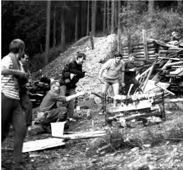
The job was completed, despite the creeping counter-revolution (photo Krkonoše National Park Administration archive)
