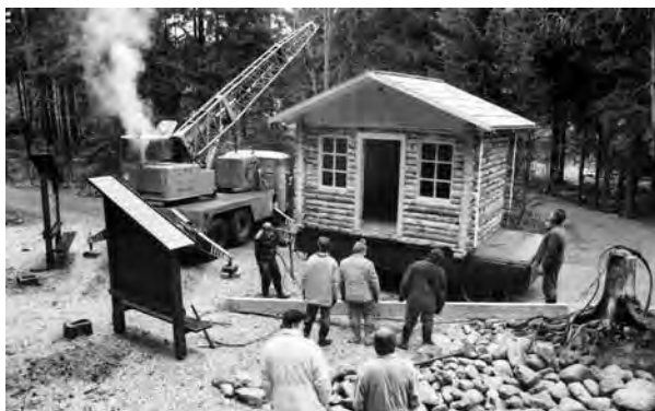
Installing the Terrain Service cabin at Dívčí lávky in October, 1994. In summer the cabin was to serve as an information point, in winter as a shelter for cross country skiers on the Keep Fit! Trail. Around the cabin are panels with educational texts, on the right the preserved roots around a spruce stump (photo Karel Hník)
